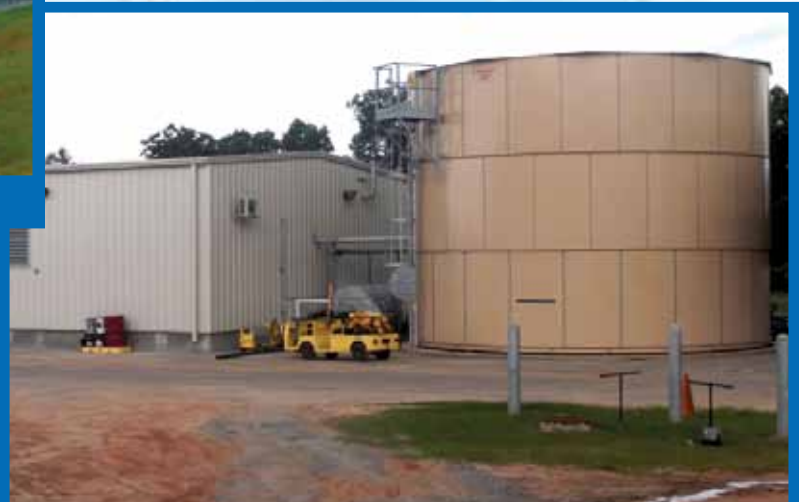
Wastewater treatment plant at Lyons, Georgia
