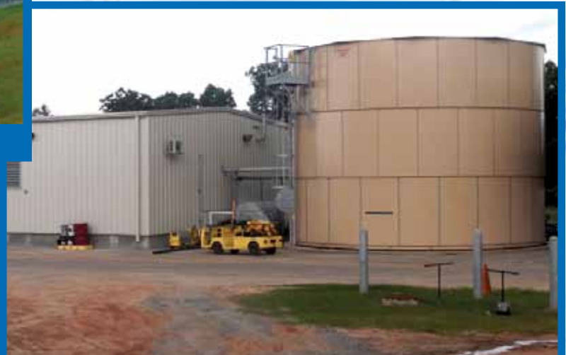
Wastewater treatment plant at Lyons, Georgia
